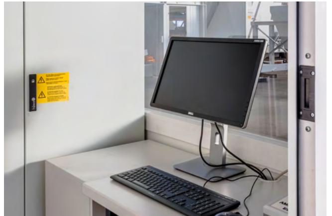
Integrated container with plant control system.
