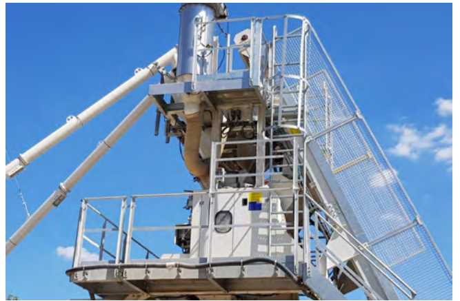
Generous service and maintenance platforms ensure best service accessibility.
