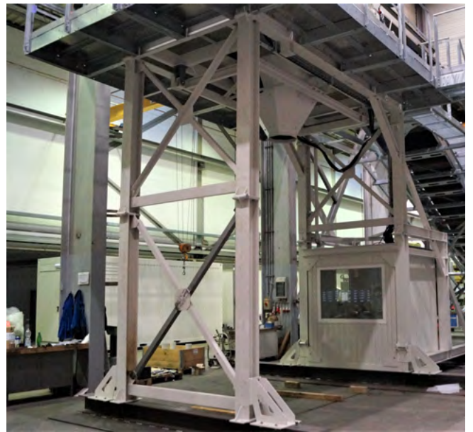
Plant structure and supports, catwalk and stairs and integrated control cabin.
