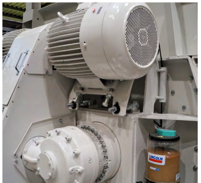
Mixer drive with automatic central greasing system.
