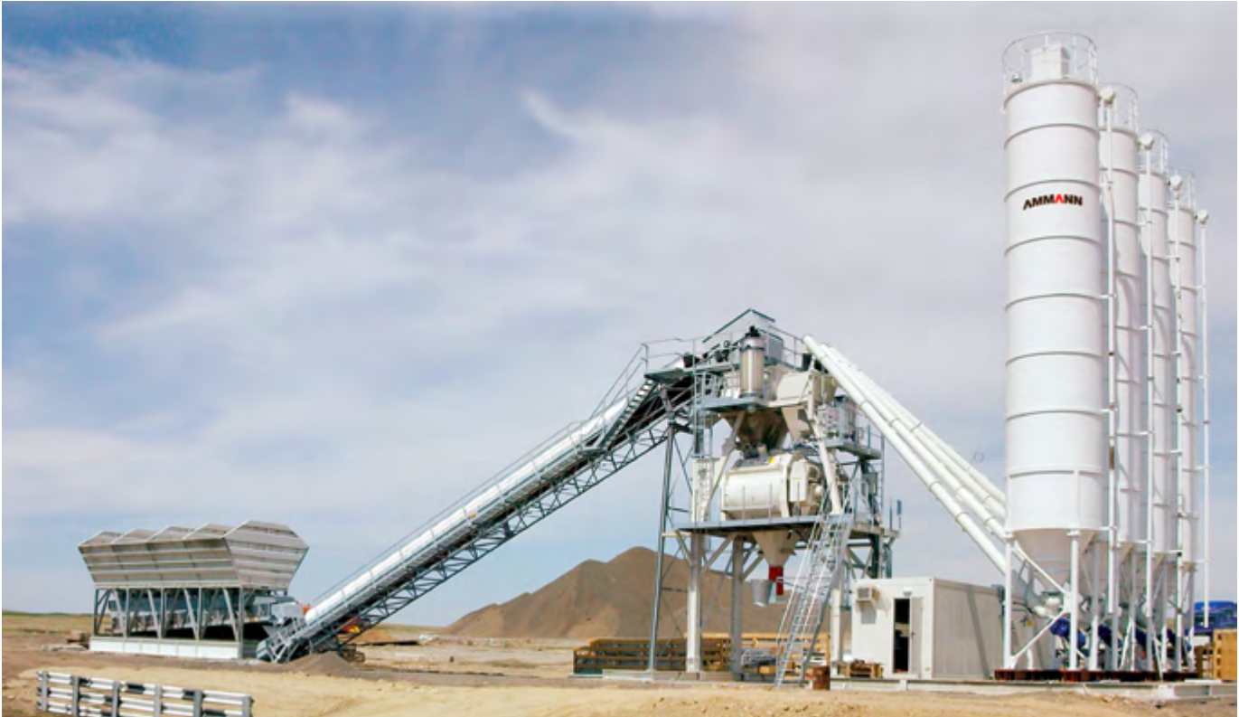
The CBS 180 TB Elba just before commissioning.
