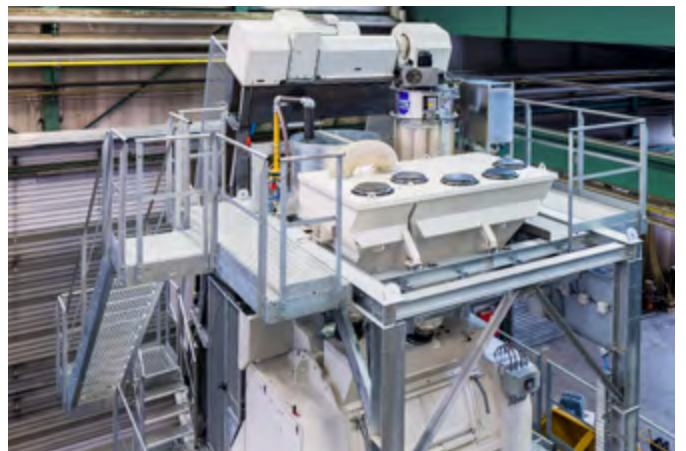
Good accessibility to the skip and weighing bin at the CBS 105 SL Elba.
